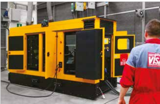
Genset soundproofed canopy
