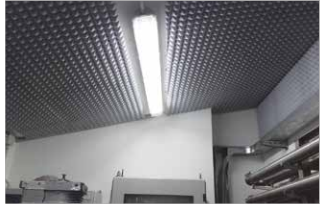
Technical room acoustic reclamation
