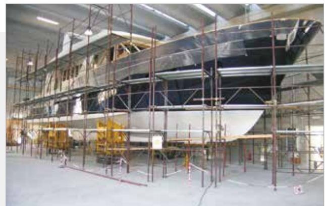
Acoustic isolation of a yacht engine compartment
