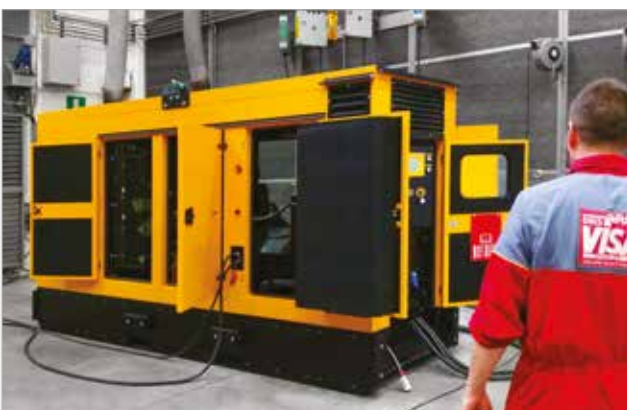
Genset soundproofed canopy
