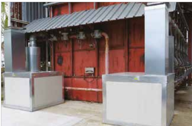
Industrial plant acoustic reclamation (enclosed fans)
