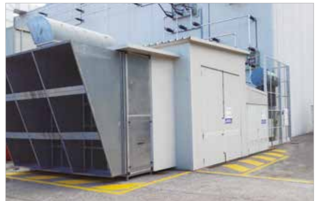
Acoustic isolation of a room housing a generating set
