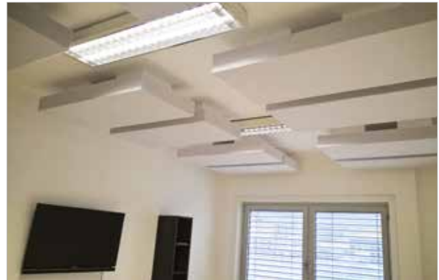
Acoustic correction inside a meeting room
