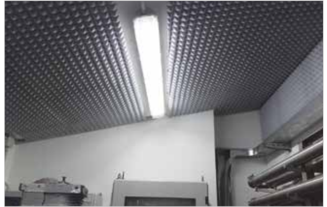
Technical room acoustic reclamation
