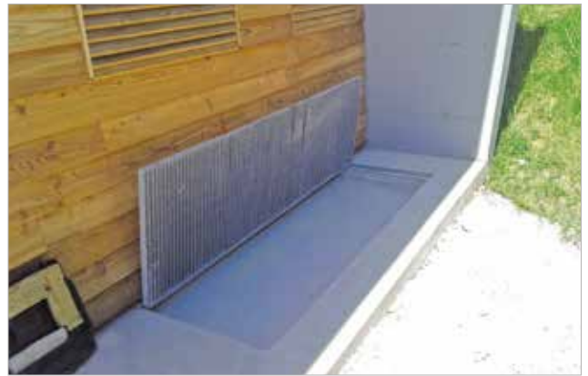
Acoustic reclamation of basement windows for hydroelectric power plants
