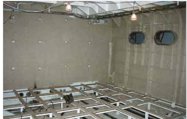
Acoustic insulation of internal wall partitions on a yacht
